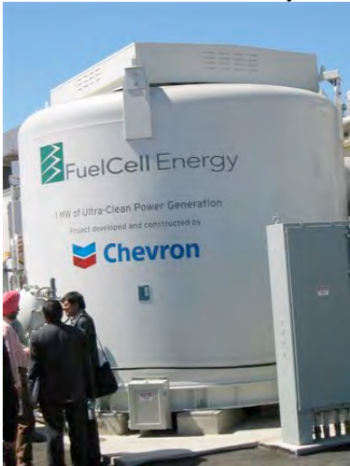
Fig. 2. The 1 MW Fuel Cell at Santa Rita Jail The fuel cell at the jail was intended to provide a consistent base load of 1 MW. The fuel cell’s performance has not been good. In fact, it produced at a 100% capacity factor in only one month over the 2007-2009 period. The missed 2009 bill savings resulting from less-than-perfect performance are shown in Figure 3.
